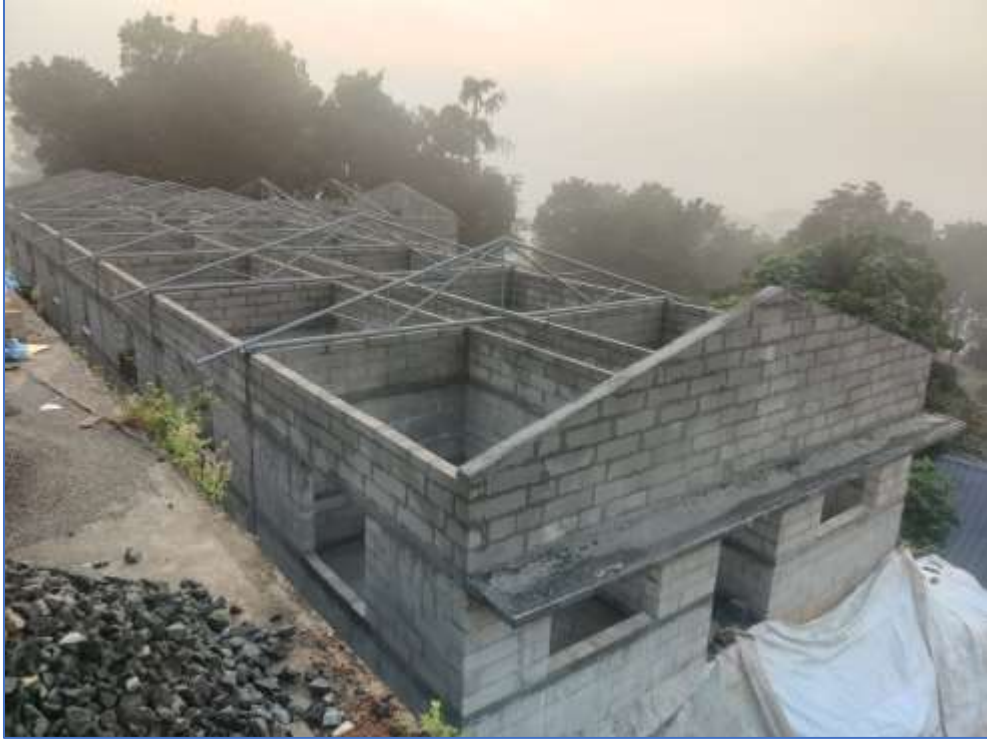
Single Storied Hostel for PhD scholars – Under construction - Through Internal Revenue Generation (IRG) (13 Dec 2023)
