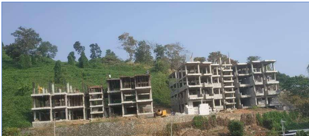
28 Staff Quarters Both the Buildings– Under Construction – Through Internal Revenue Generation (IRG) (on 03 Jan 2023)
