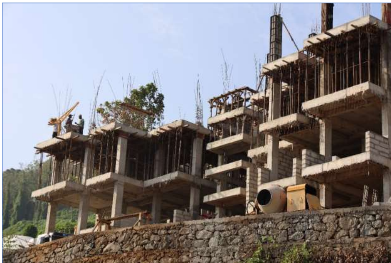
28 Staff Quarters 1 st Building – Under Construction – Through Internal Revenue Generation (IRG) (on 05 Feb 2024)
